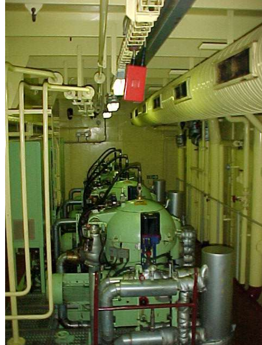
Detection in Main Engine Room
