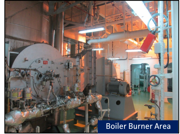
Boiler MDO Supply Pumps
