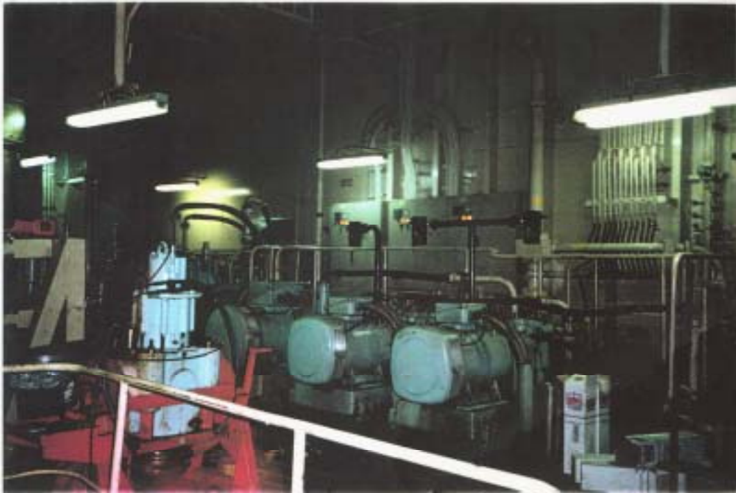
Protection of Compressors and Pumps
